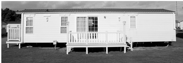
Does not meet standard for skirting.
